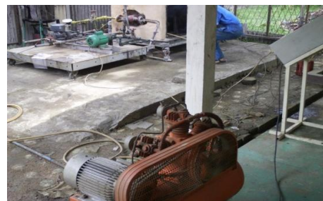
Gambar 5. Compressor, Electrical Panel on-off, Fuel Oil Pump, Steam Product Flow Meter dan Fuel Oil Tank
