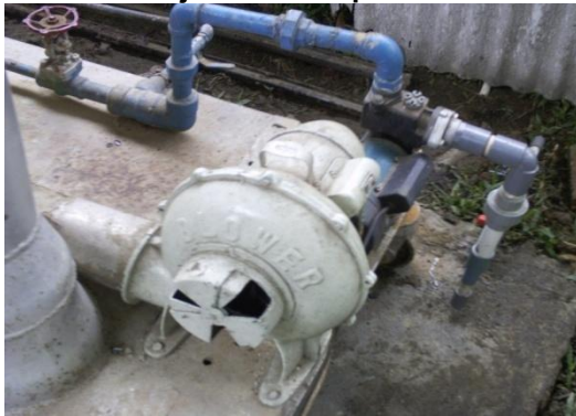
Gambar 8. Cerobong Asap, Blower dan Boiler Feed Water Pump
