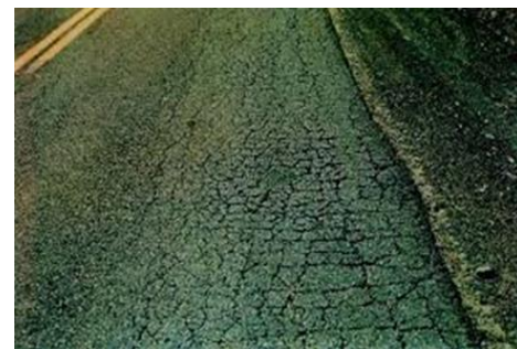
1.d. Alligator cracking
