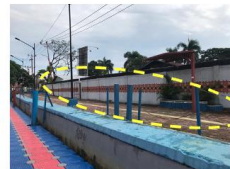
(c) Tiang-tiang hilang
